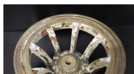
Image – cage surface corrosion can be sanded or blasted off before reassembly
